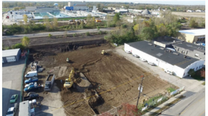
1123 Goodale after demolition of original 1940 building; Goodale Boulevard is at the bottom right, and the City of Columbus Dublin Road Water Plant is at the top left.
